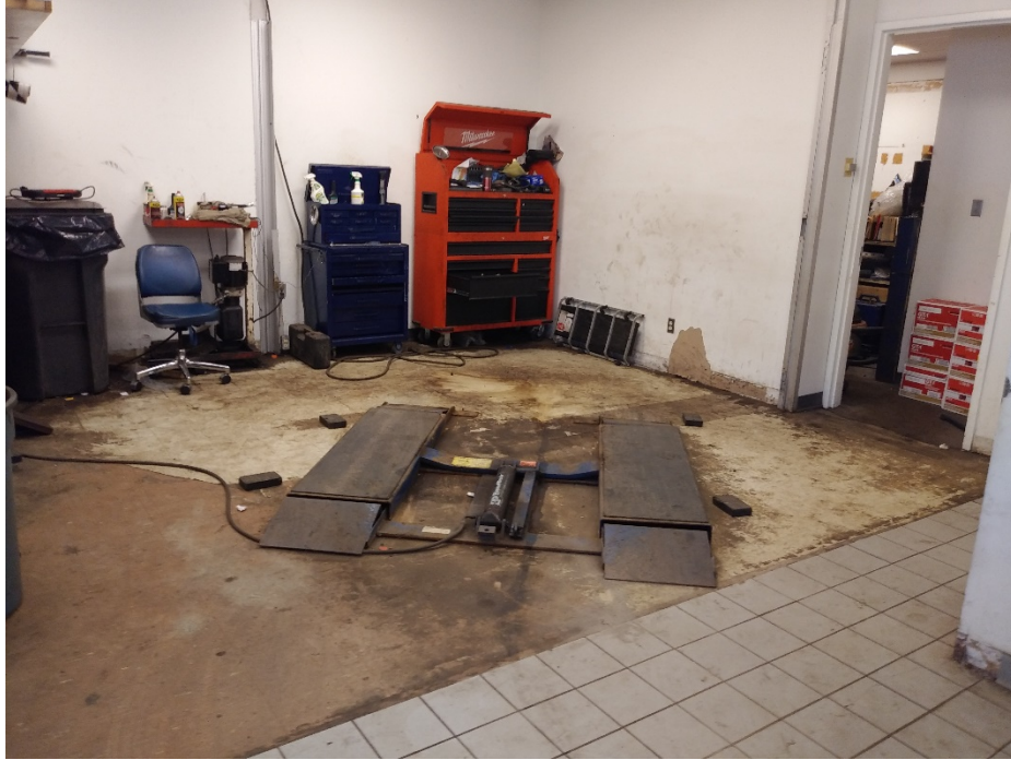
Photograph 7: View of the interior of the automotive service garage in the south unit of the south commercial building. View shows an aboveground hoist and some equipment storage.
