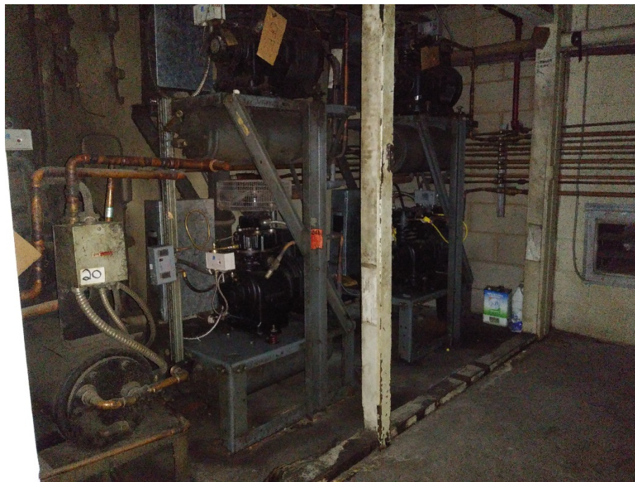
Photograph 10: View of the refrigeration equipment in the penthouse level of the former grocery store in the northwest portion of the north commercial plaza building.
