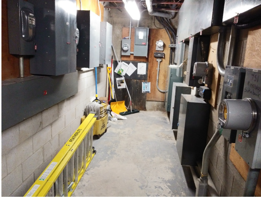
Photograph 9: View of the basement electrical room in the north commercial plaza building.
