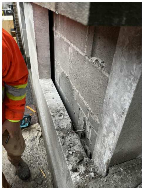
Figure 12: View of a test removal panel from a building at 100 Argyle constructed circa 1955 using a similar limestone cladding material as 359 Kent. The limestone cladding units are secured to the concrete block back-up wall with a single metal anchor centred on the width of the panel. Source: Heritage Grade Test Removal Report, 100 Argyle.
