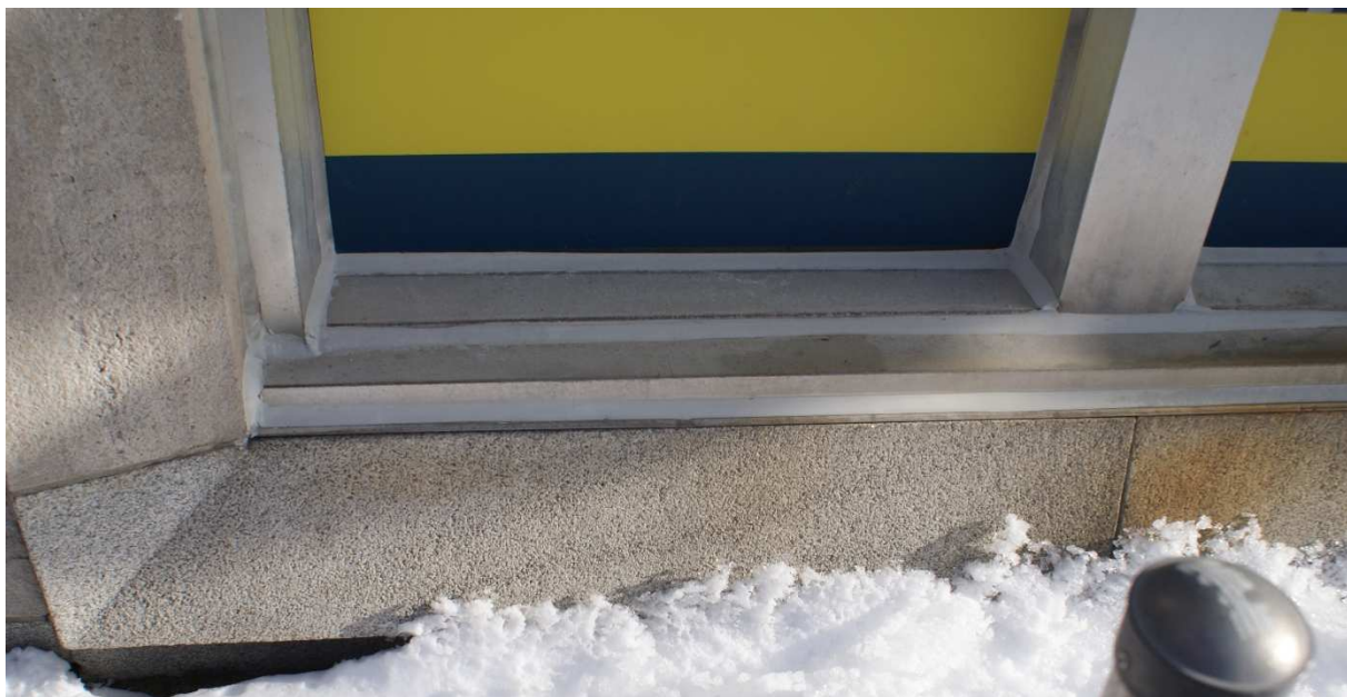
Figure 23: Detail view of the base of the Kent Street window. The horizontal units at the base of the window are formed of the same material as the granite plinth course. The vertical stone to the left is a limestone unit. Note the close match in colour and surface texture. Source: Commonwealth 2023
