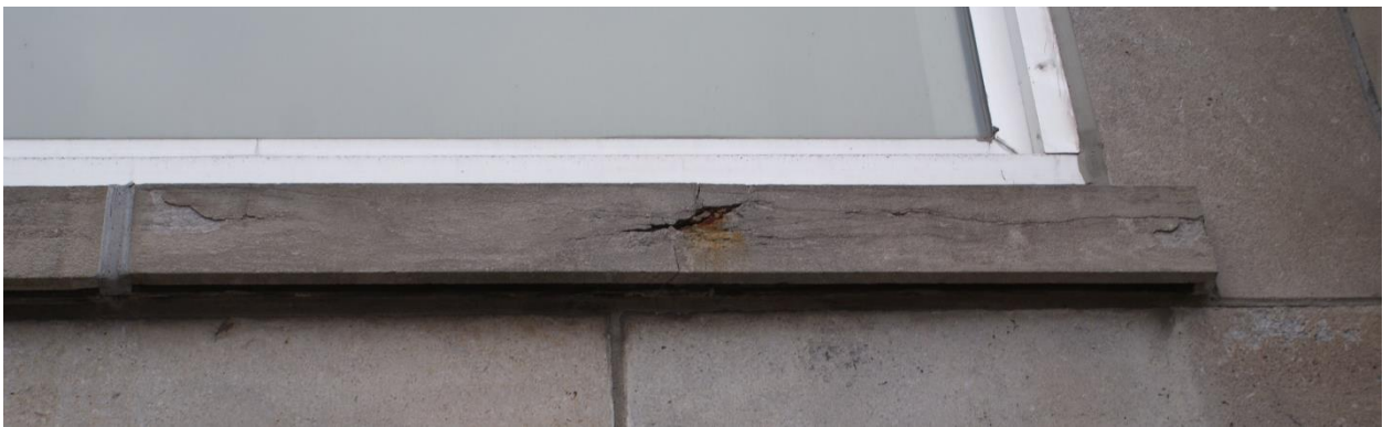
Figure 14: View of a deteriorated limestone windowsill. The cleavage planes within the limestone sills are evident where the sawn surface. The cleavages follow the layers of deposition of the sedimentary rock. Source: Commonwealth 2022.
