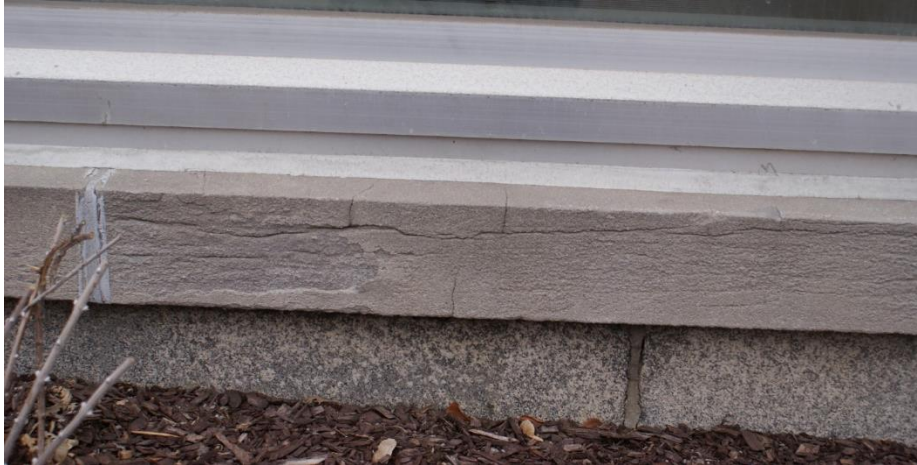
Figure 13: View of a deteriorated limestone windowsill and the granite plinth course below. The cleavage planes within the limestone sills are evident where the sawn surface has weathered. The cleavages follow the layers of deposition of the sedimentary rock. Source: Commonwealth 2022.
