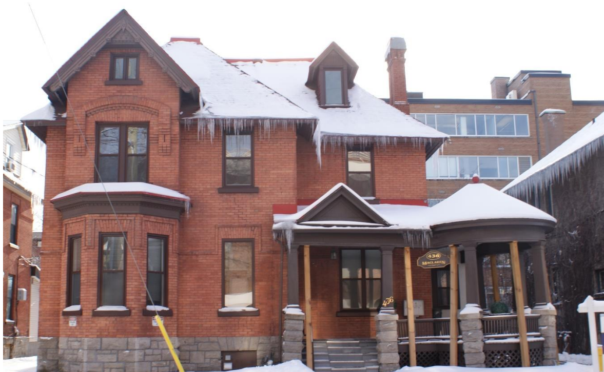
Figure 25: View of 436 MacLaren Street. The masonry piers supporting the porch have settled due to inadequate foundation depth. A detailed assessment of the condition of the porch is required. Guidelines from the CHCDP provide guidance for the conservation approach to the materials and assemblies. Source: Commonwealth 2023.
