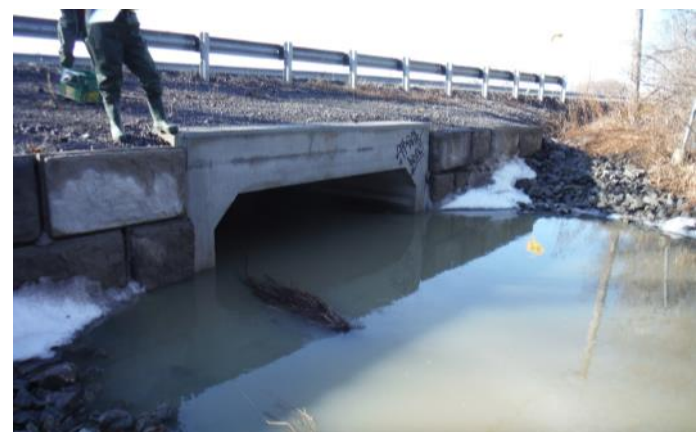
Channel hardening at an HDF site along Corkstown Road
