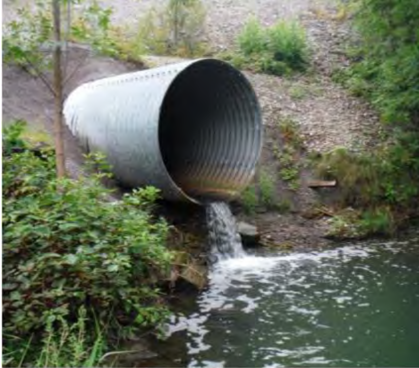
Figure 1: Photo of perched culvert that conveys flow of Stillwater Creek under the Beachburg Rail line (RVCA, 2015)
