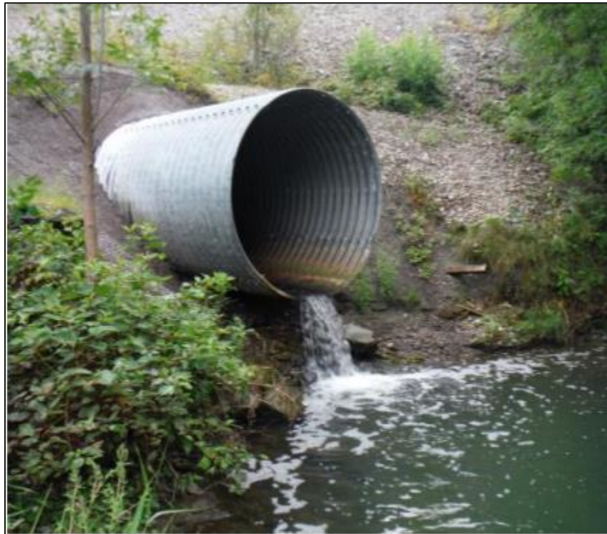
Photo 1: Perched culvert that conveys flow of Stillwater Creek under the Beachburg railway (RVCA, 2015)
