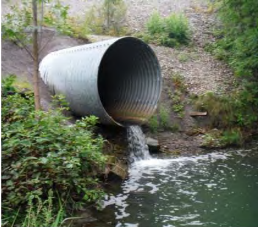
Figure 1: Photo of perched culvert that conveys flow of Stillwater Creek under the Beachburg Rail line (RVCA, 2015)
