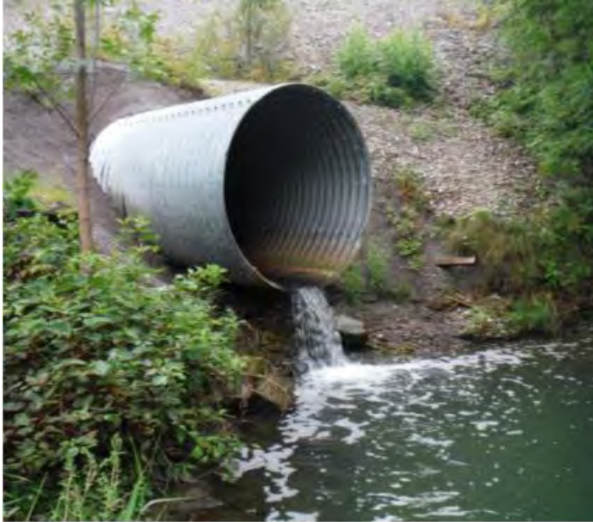
Figure 3: Photo of perched culvert that conveys flow of Stillwater Creek under the Beachburg railway (RVCA, 2015)
