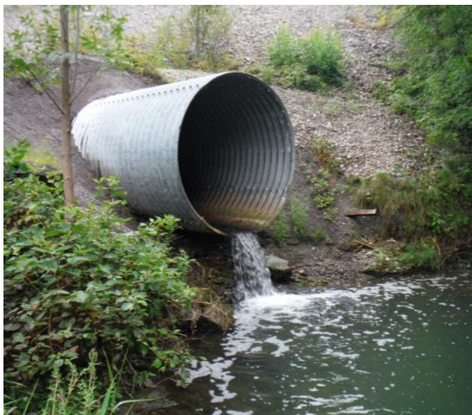
A perched culvert observed along a tributary of Stillwater Creek
