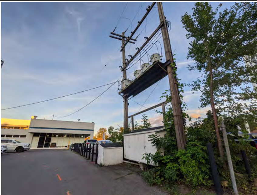
Photo 11 - Suspended transformers, westside parking lot entrance, adjacent to New Orchard Ave, facing northeast
