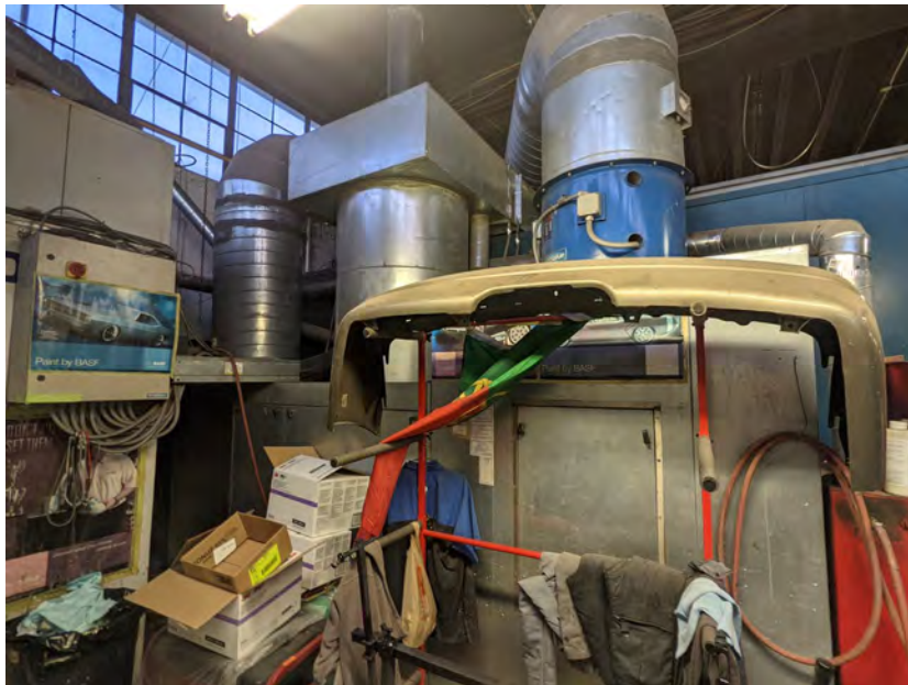
Photo 28 – Exhaust for the paint booth
