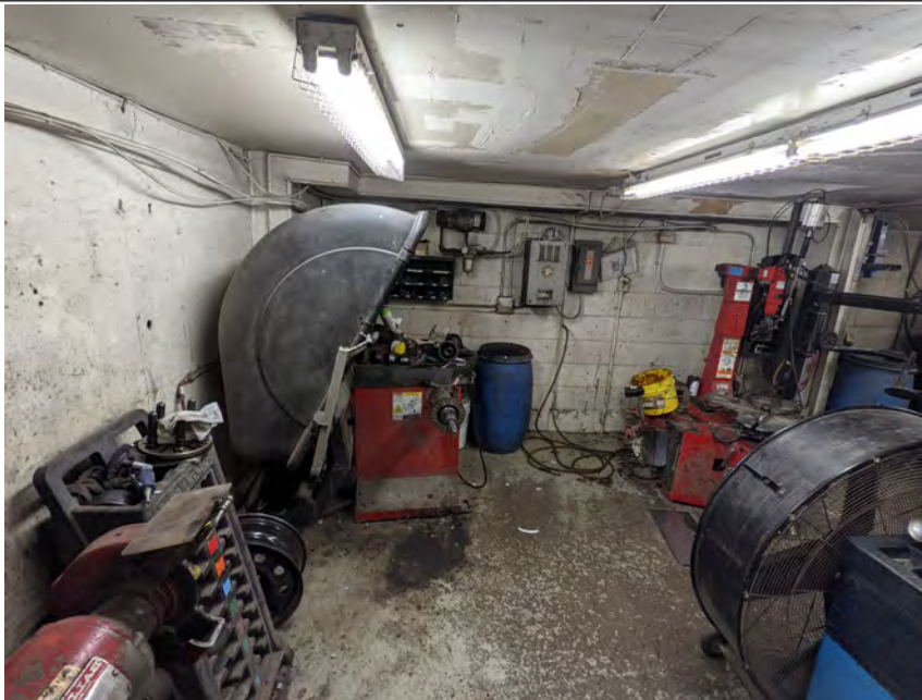
Photo 25 – Tire balancing machine, eastside of the garage
