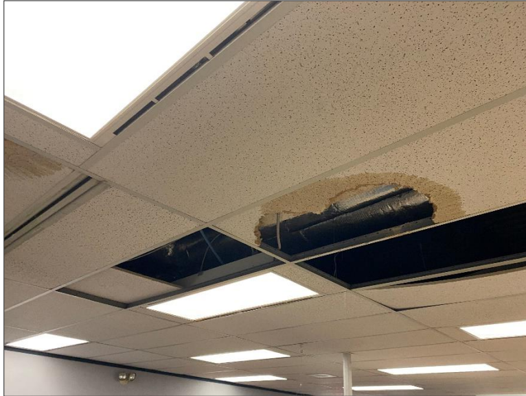
Photo 9 – Stained ceiling tiles located within the office portion of the Site Building.
