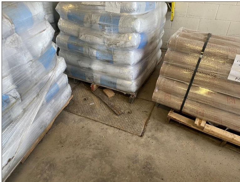
Photo 12 – OWS located within the southwest portion of the Site Building.
