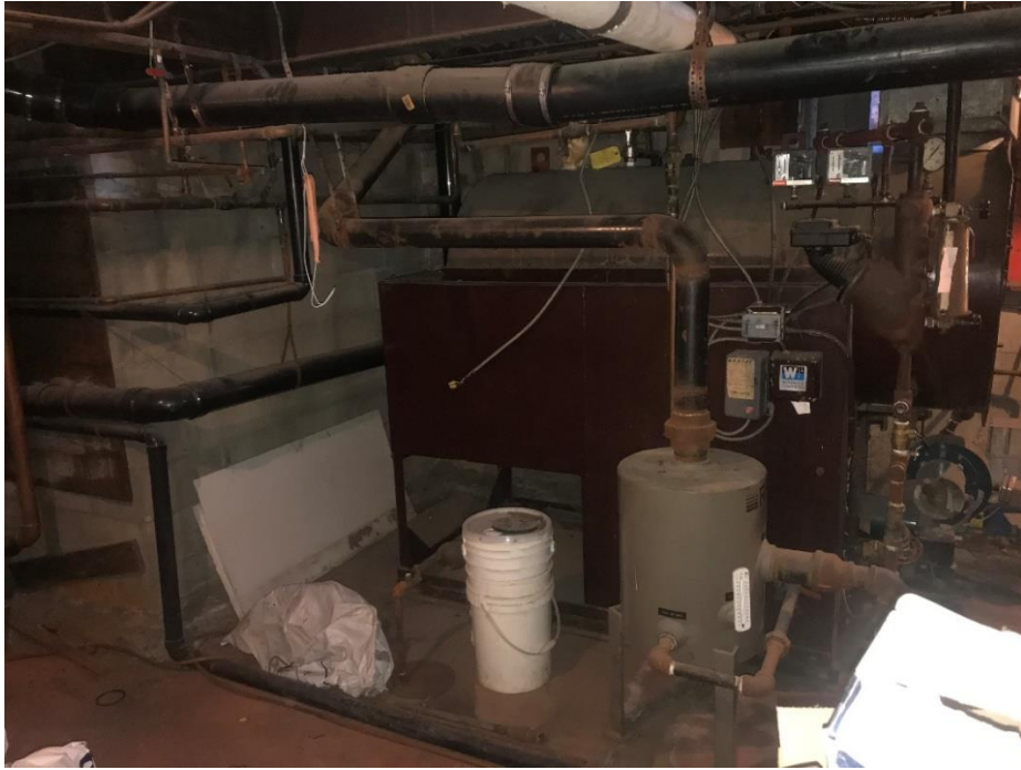
Photograph 27: Boiler in basement of Site building (April 6, 2021).
