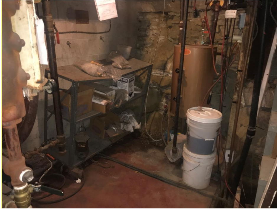
Photograph 29: Boiler blow down tanks in basement of Site building (April 6, 2021).
