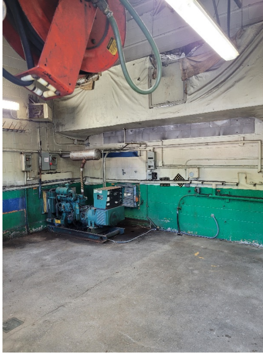
Photograph 5: View of the interior of the service bay, on the east portion of the Property. The diesel generator is visible in this photograph.
