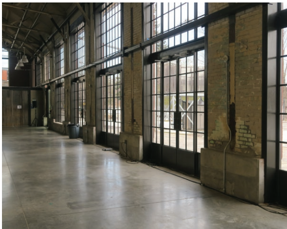
Deteriorating brick walls on the east interior elevation of the exhibition hall (ERA 2023)
