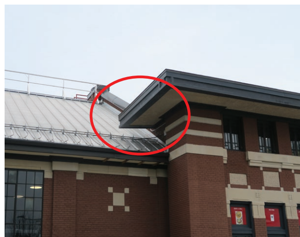
Sagging corner of the flat roof on the northwest corner of the entrance hall (ERA 2023)
