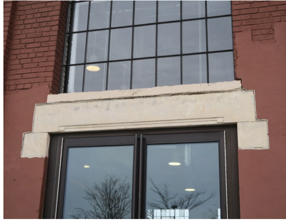
Delaminated and cracked stone sill and header on east elevation of exhibition hall (ERA 2023)
