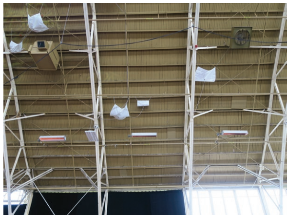
Wood roof purlins and decking. Note gaps between wood decking and rain capture tarps (ERA 2023)
