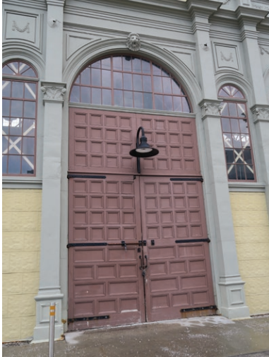
North entrance pavilion doors. Areas of dry/split wood and gaps are noted (ERA 2023)
