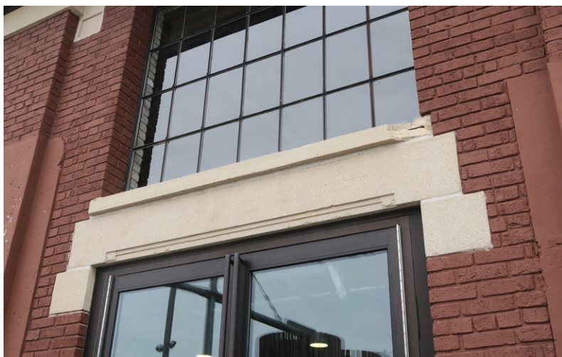
Chipped stone sill above door on east elevation of the exhibition hall (ERA 2023)
