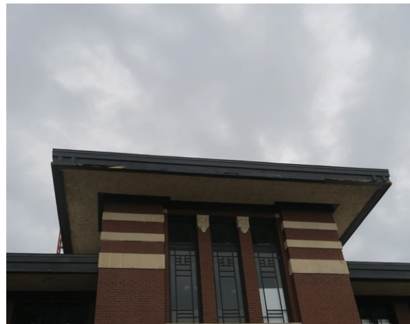
Chipped wood fascia on south elevation flat roof (ERA 2023)
