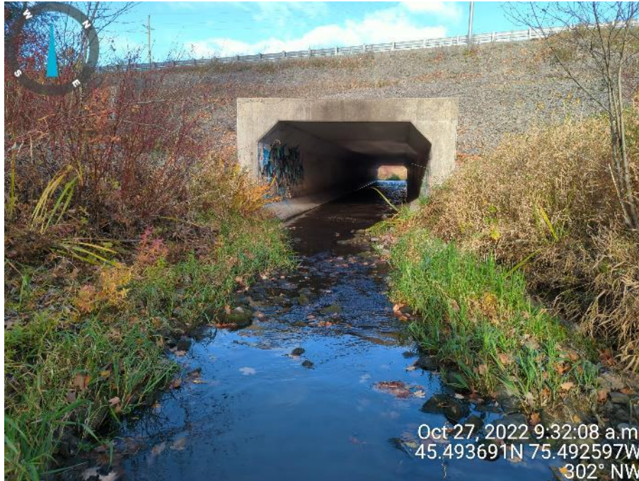
Photo 9: Taylor Creek downstream end, looking downstream at the culvert flowing under Jeanne d'Arc Boulevard North (October 27, 2022)
