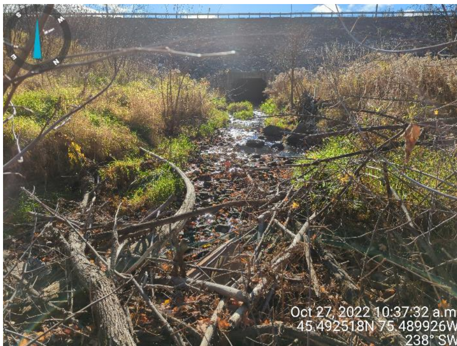
Photo 12: Taylor Creek near the upstream end, looking upstream at the culvert flowing under Highway 174 (October 27, 2022)
