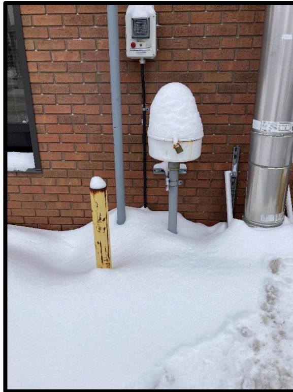
Photograph 3: View of the vent and fill pipes along the back wall of the 50 Bayswater Avenue office building, facing east.
