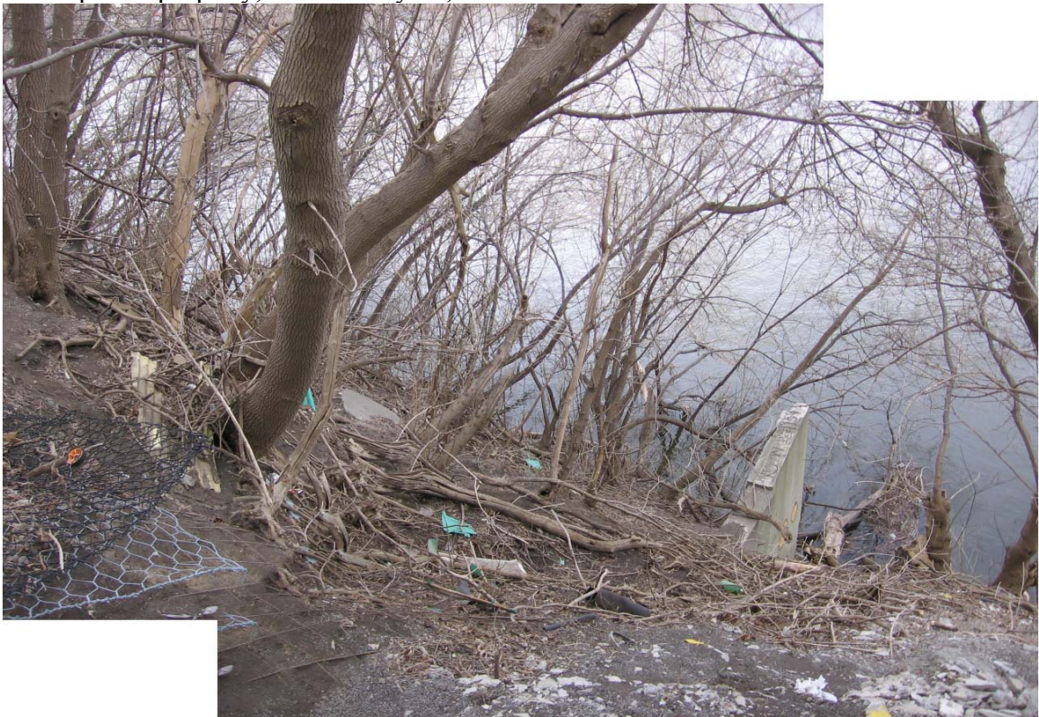
Photo 4. View down slope to the Rideau River on March 25, 2010. The concrete abutment is the upstream extent of the development property.
