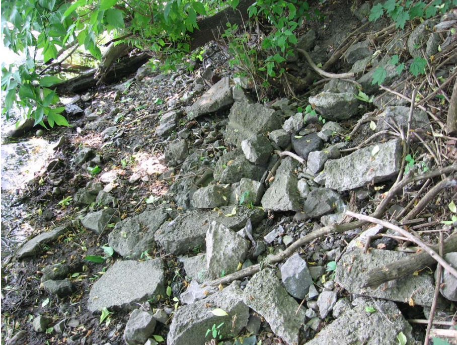
Photo 12. Shoreline showing broken concrete that has been moving downslope toward the river – May 25, 2010.
