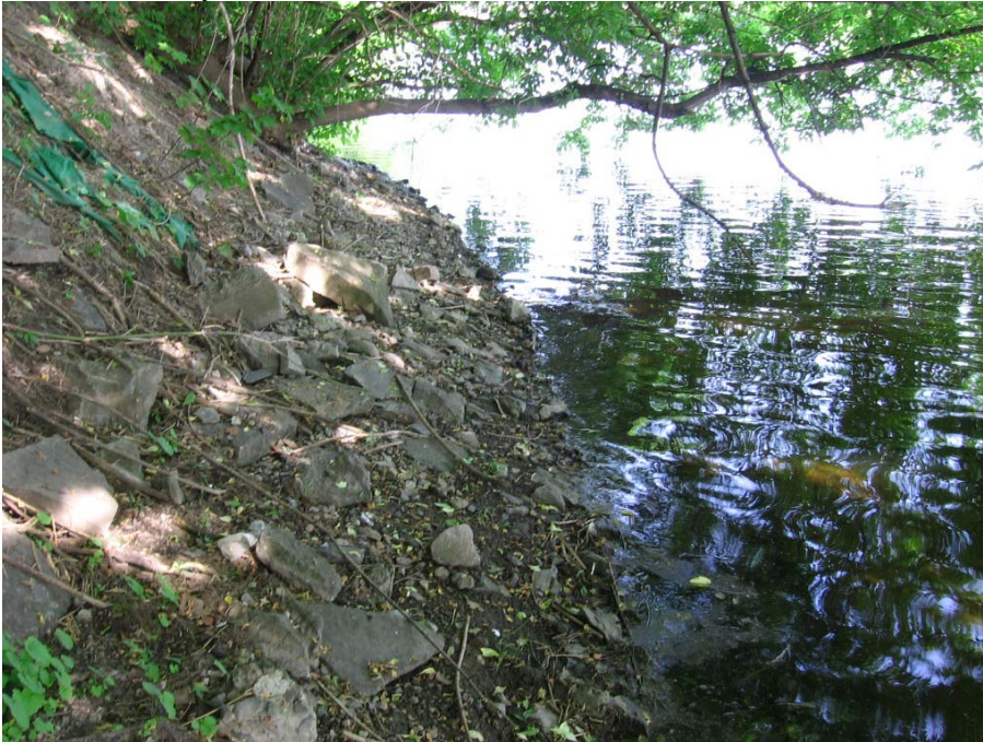
Photo 13. Shoreline showing broken concrete and unconsolidated material that has been moving downslope toward the river. While the Manitoba maples provide overhead shade, the shoreline itself lacked riparian vegetation – May 25, 2010.
