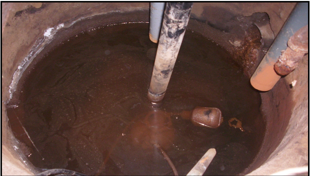
Photograph 6: Sump pit in boiler room.
