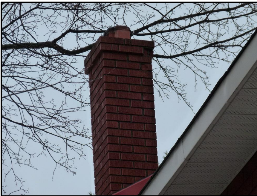
Photograph 6: Chimney #3 at 540 Edison Avenue. Note ceramic liner with wire mesh cap (March 28 th , 2017).
