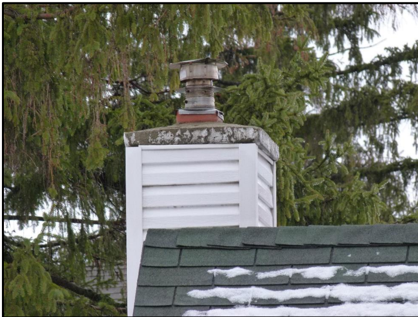
Photograph 2: Chimney #1 at 530 Edison Avenue. Note metal cap and ceramic liner (March 28 th , 2017).
