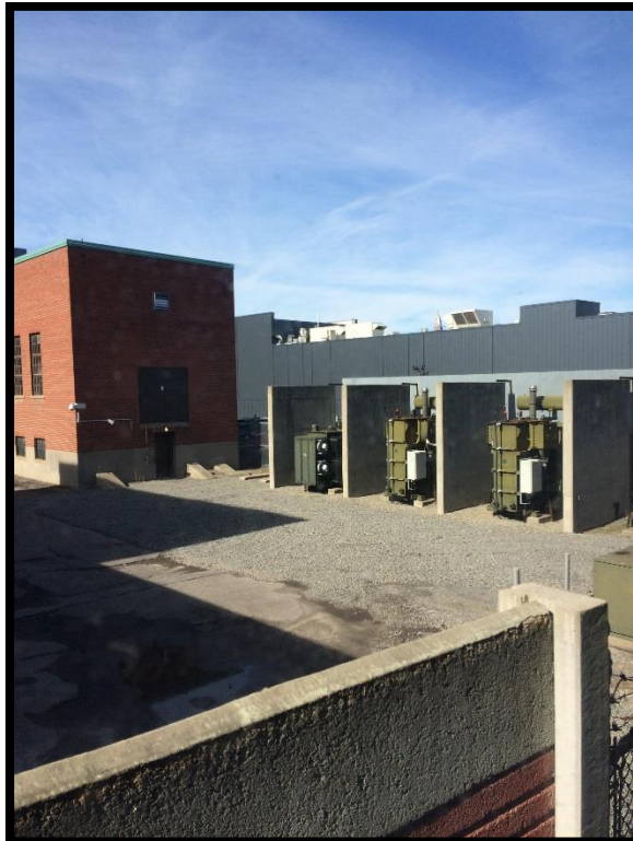
Photograph 6: View of the adjacent transformer substation, looking northwest.
