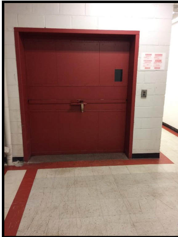
Photograph 4: Cable operated freight elevator within central area of the building.
