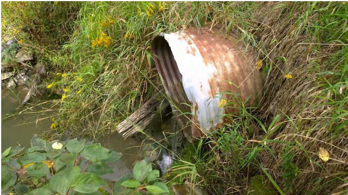
Photograph No. 2: View of south end of culvert under the roadway (Location 2 on Figure 2)
