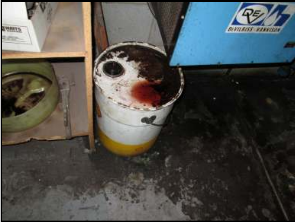
Photograph 5: Hydraulic oil and minor staining on floor slab in penthouse mechanical room.
