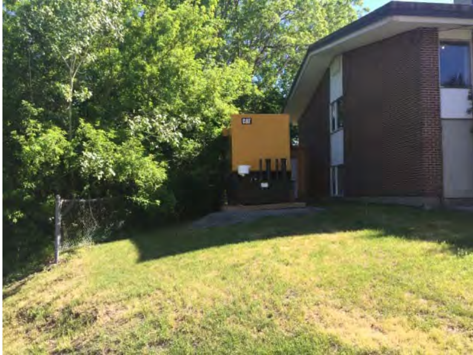
Photo 5: Diesel generator with an associated AST located on the north side of the nursing home at 99 New Orchard Avenue.
