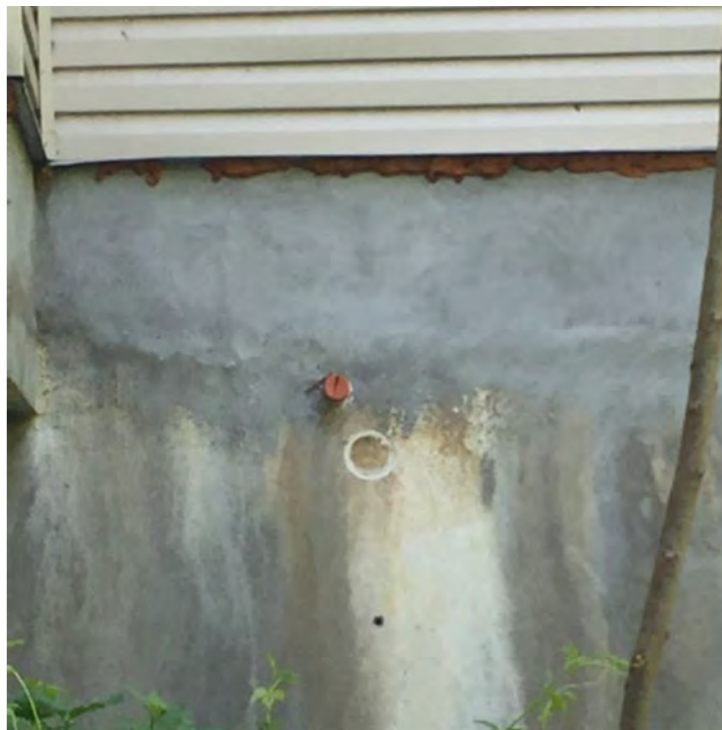
Photo 2: Photo of the pipe and filled in hole of a former pipe located in the basement foundation on the on-Site residential building. They are likely former fill and vent pipes for a former heating oil AST.
