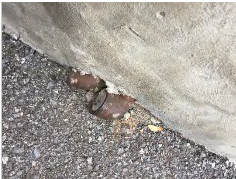
Photo 6 – Inferred vent/fill pipes for an AST located at 171 George Street (approximately 15 m northeast of the Phase One Property).
