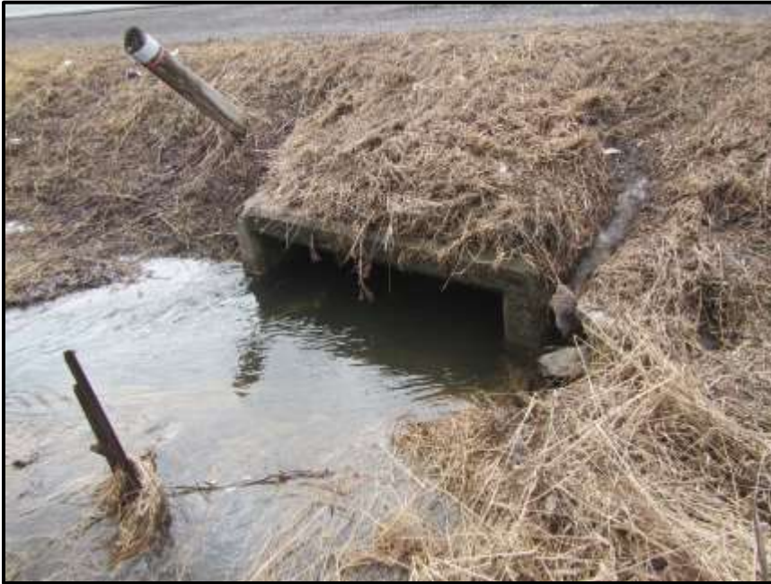
Photograph 3: Survey Site #1 - 2 m concrete box culvert under March Road (facing upstream) (March 30 th , 2018).
