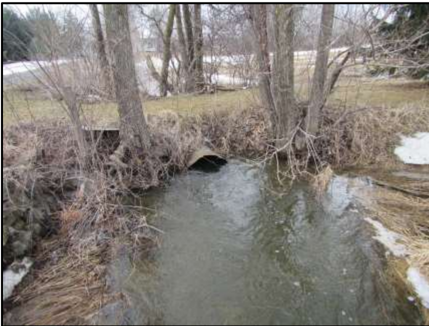
Photograph 4: Survey Site #1 - 60 cm CSP culvert under the driveway west of March Road (facing upstream) (March 30 th , 2018).
