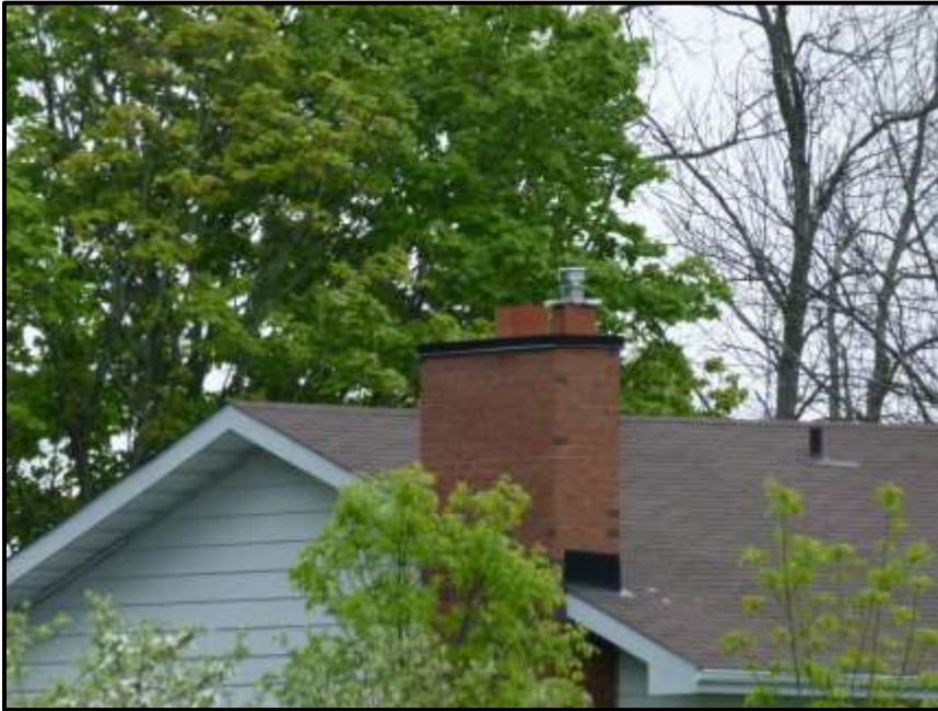
Photograph 35: Chimney at 1145 March Road. Note the ceramic liner and metal cap (May 24 th , 2017).
