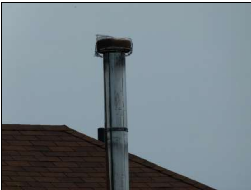
Photograph 34: Chimney at 1113 March Road. Note the metal liner and wire mesh cap (May 24 th , 2017).
