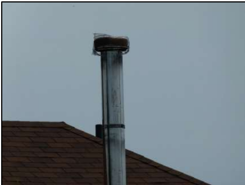
Photograph 34: Chimney at 1113 March Road. Note metal liner and wire mesh cap (May 24 th , 2017).
