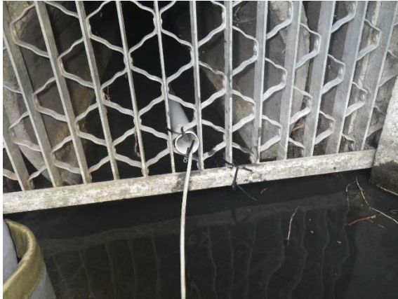
Figure 2a: Stingray and water level logger Installation on culvert grate at Q1
