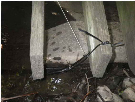
Figure 2c: Water level logger installation at Q3
