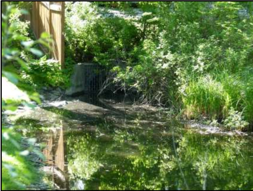
Photograph 109: Pipe from the adjacent subdivision that feeds water into the Stormwater Infiltration Swale within Section #5 (May 24 th , 2018).
