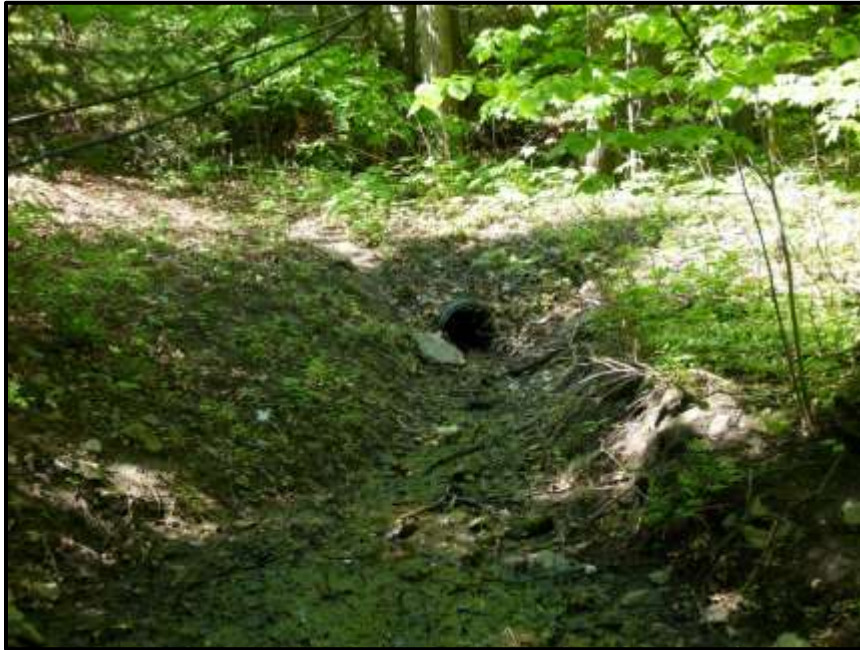
Photograph 111: Pipe from the adjacent subdivision that feeds water into the Stormwater Infiltration Swale within Section #6 (May 24 th , 2018).
