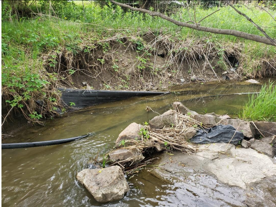
Exposed filter cloth and bank erosion adjacent to exposed bedrock along the right bank. At this location, it is assumed that the presence of bedrock increases channel energy to the left bank.
