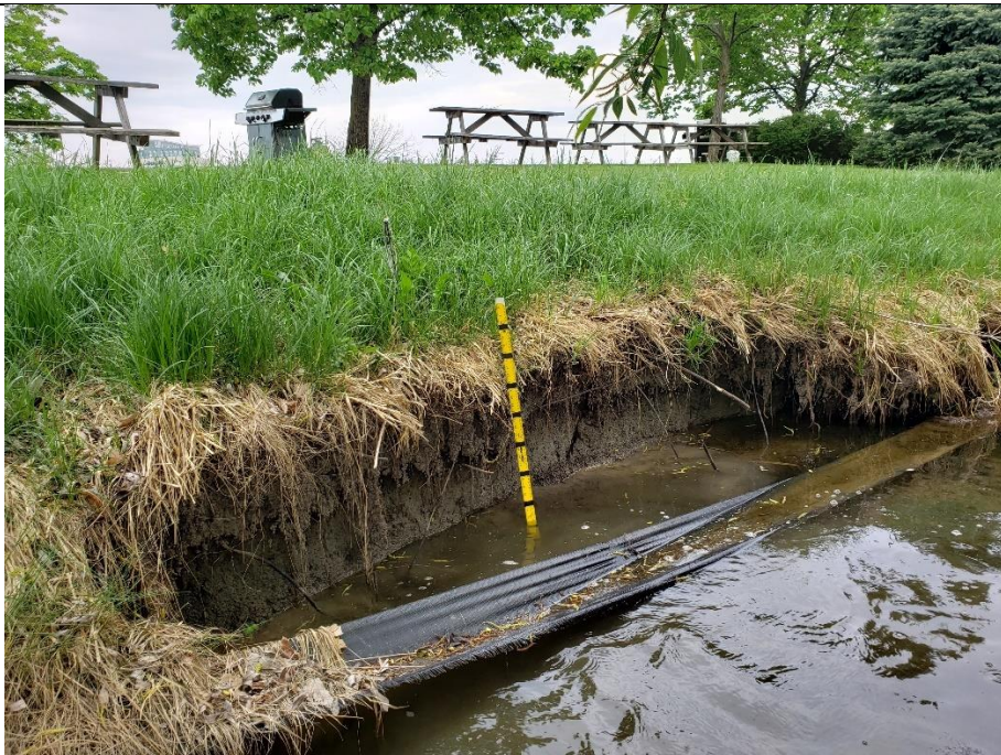
In this instance of bank erosion, the riparian vegetation has been cut and maintained. The lack of riparian vegetation and rooting structure is assumed to have resulted in the increased erosion.
