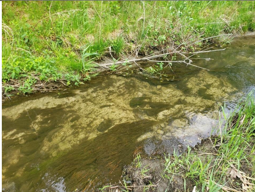
Downstream of the armoured section near the pedestrian bridge, exposed compact clay was observed. This material was consistently observed as the underlying material throughout Kizell Drain.
