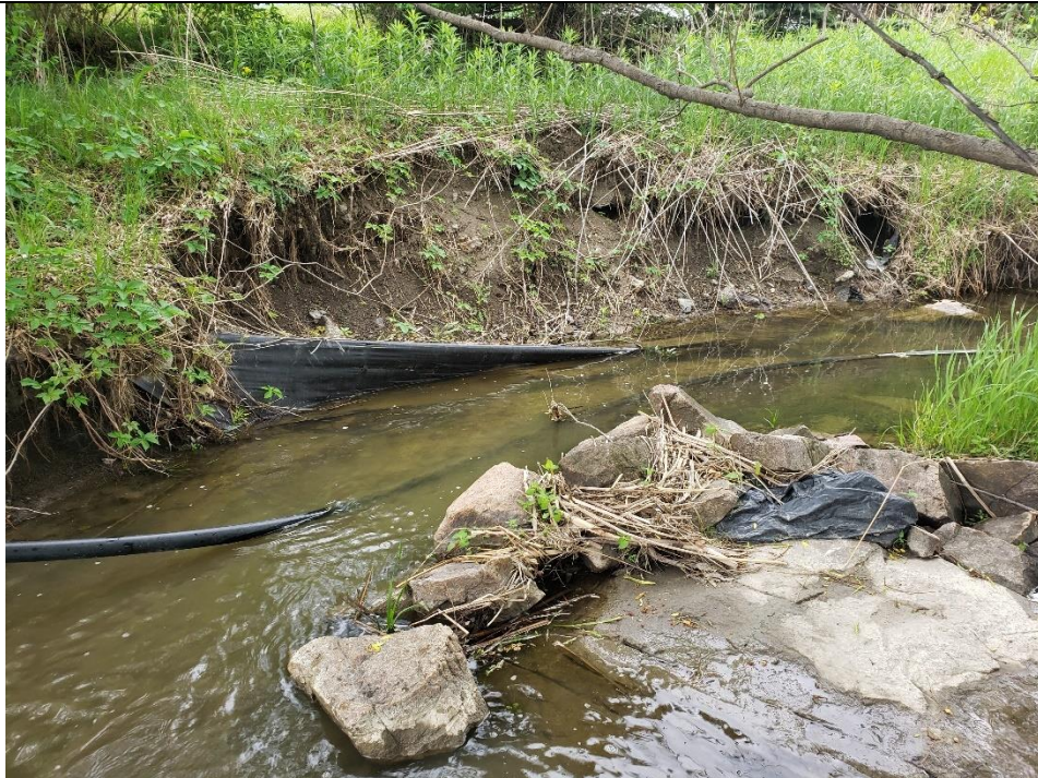
Exposed filter cloth and bank erosion adjacent to exposed bedrock along the right bank. At this location, it is assumed that the presence of bedrock increases channel energy to the left bank.
