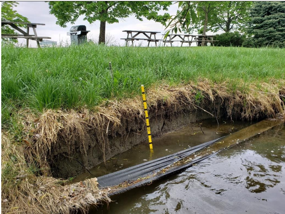
In this instance of bank erosion, the riparian vegetation has been cut and maintained. The lack of riparian vegetation and rooting structure is assumed to have resulted in the increased erosion.
