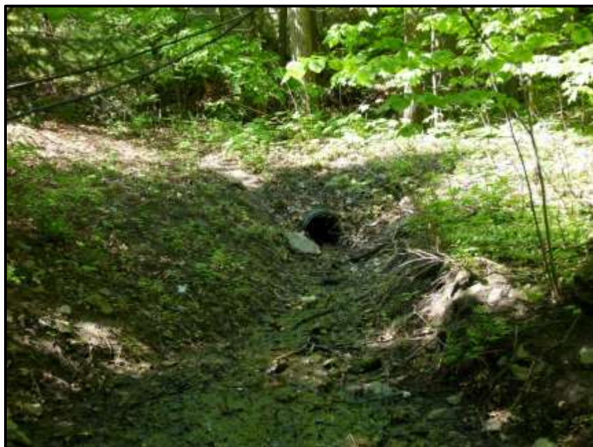
Photograph 111: Pipe from the adjacent subdivision that feeds water into the Stormwater Infiltration Swale within Section #6 (located north of the clubhouse) (May 24 th , 2018).
