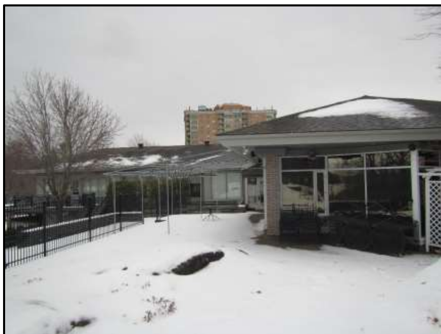
Photograph 146: Looking south at Building #3. No significant exterior openings were noted (January 10 th , 2020).
