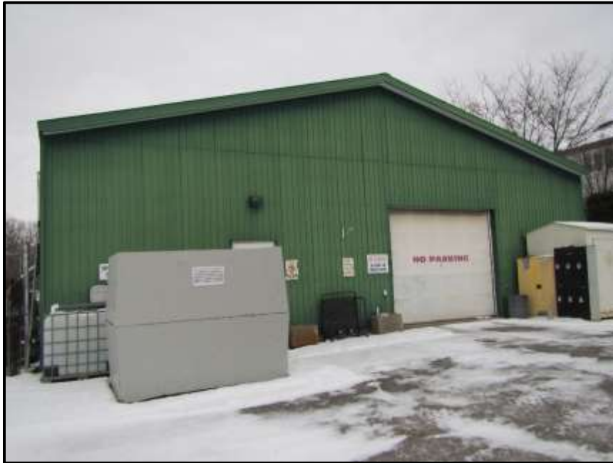
Photograph 142: Looking east at Building #1. The garage door is closed on a nightly basis. No significant exterior openings were noted (January 10 th , 2020).
