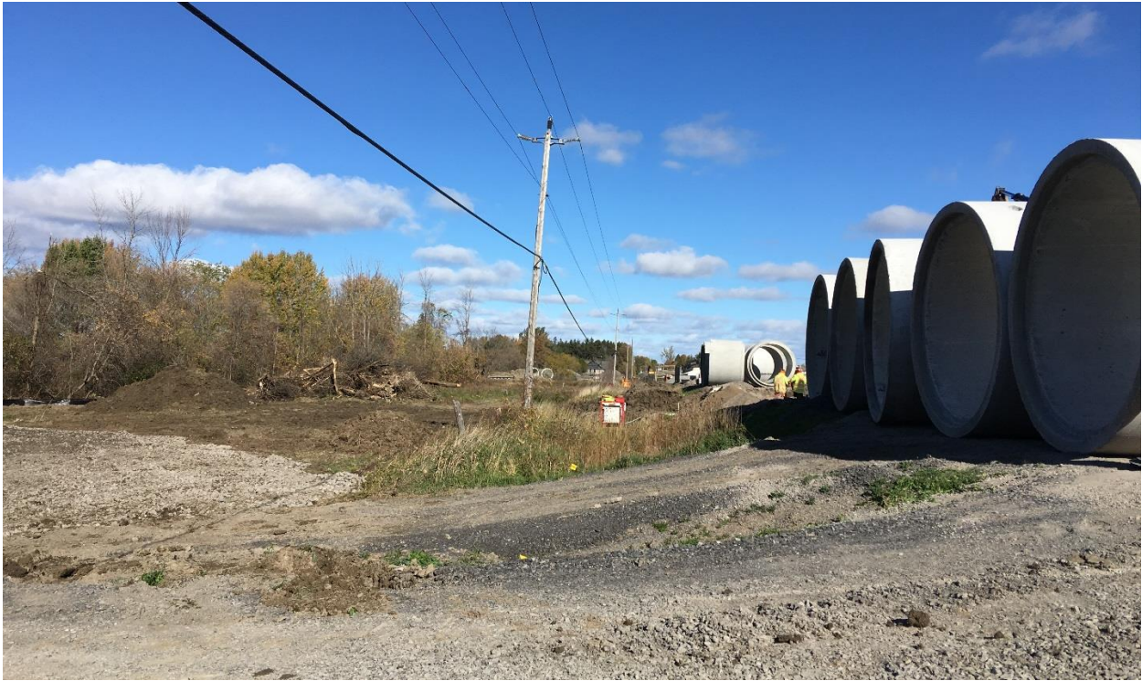
Photograph 3: View of the northeast side of the subject site, along River Road, looking north.
