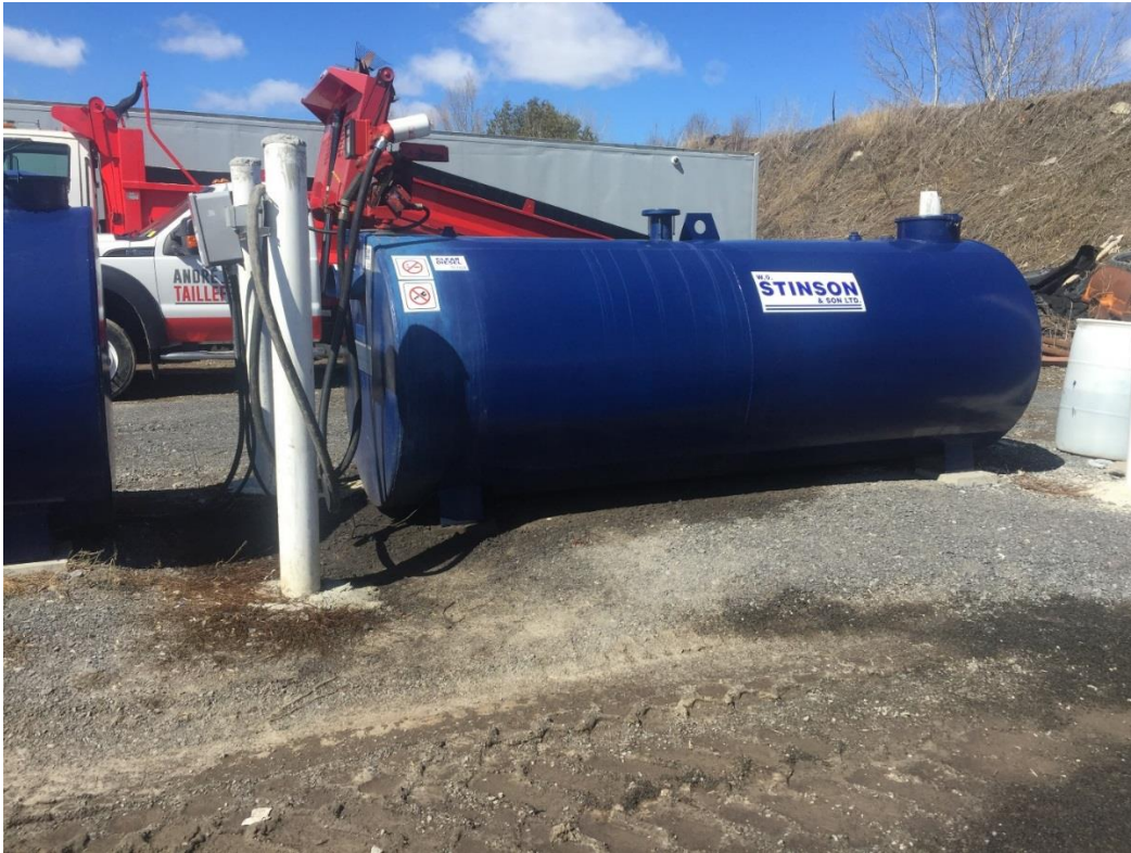
Photograph 7: Staining below the AST
