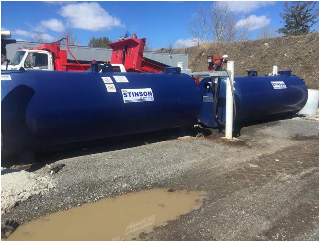
Photograph 6: Two above ground diesel storage tanks
