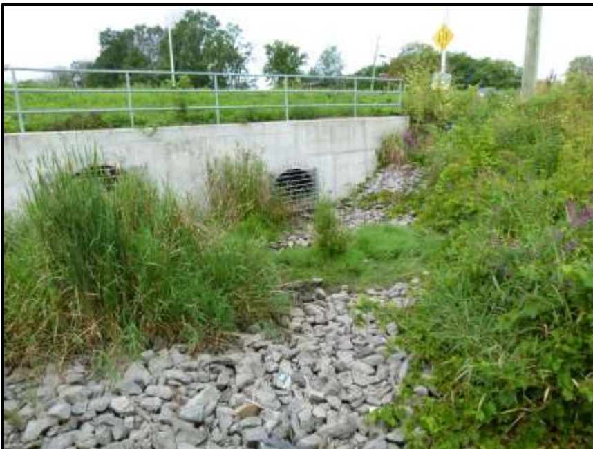
Photograph 15: Stormwater pipes outletting to the southern stormwater swale (Tributary #4) (facing west towards March Road). Note the lack of surface water (August 14 th , 2017).
