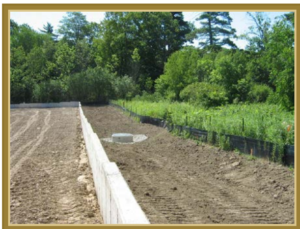
Plate 6. Stand-alone continuous concrete wall used to exclude salamander species installed as pre-cast forms (photo credit: Steven Roorda).
