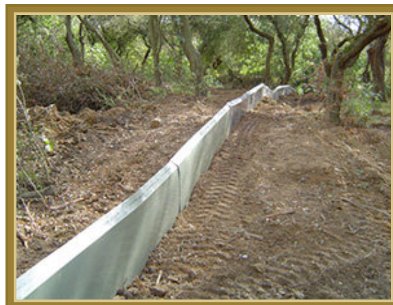
Plate 7. Pre-formed vinyl sheeting fence intended to exclude salamanders for a construction site (photo credit: Herpetosure Ltd.)
