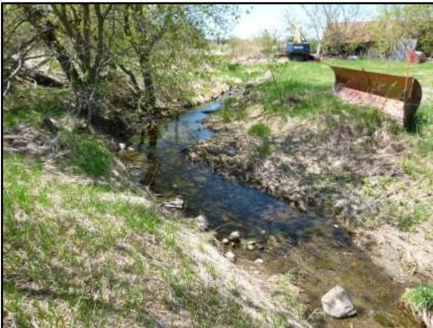
Photograph 11: Looking north along the North Branch in the eastern portion of the Site. The collapsing barn is shown in the background (May 12 th , 2018).
