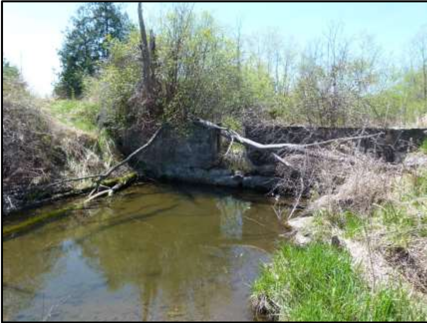
Photograph 14: Looking west at the concrete weir (west of the inline pond) (May 12 th , 2018).
