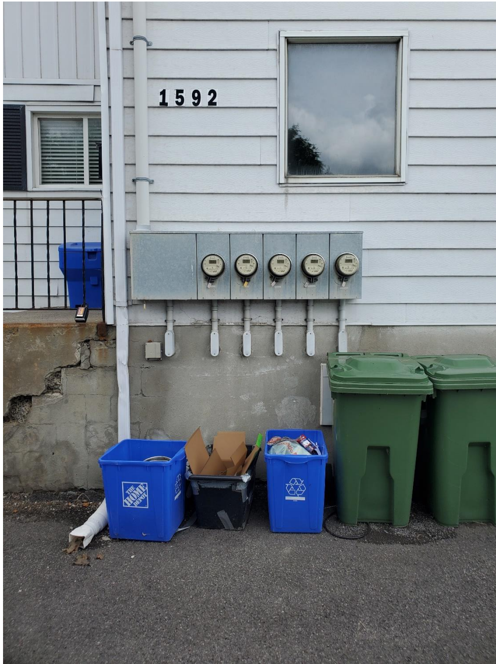
Photo 3: Facing south, overhead hydrolines enter the property from the south side of the building.
