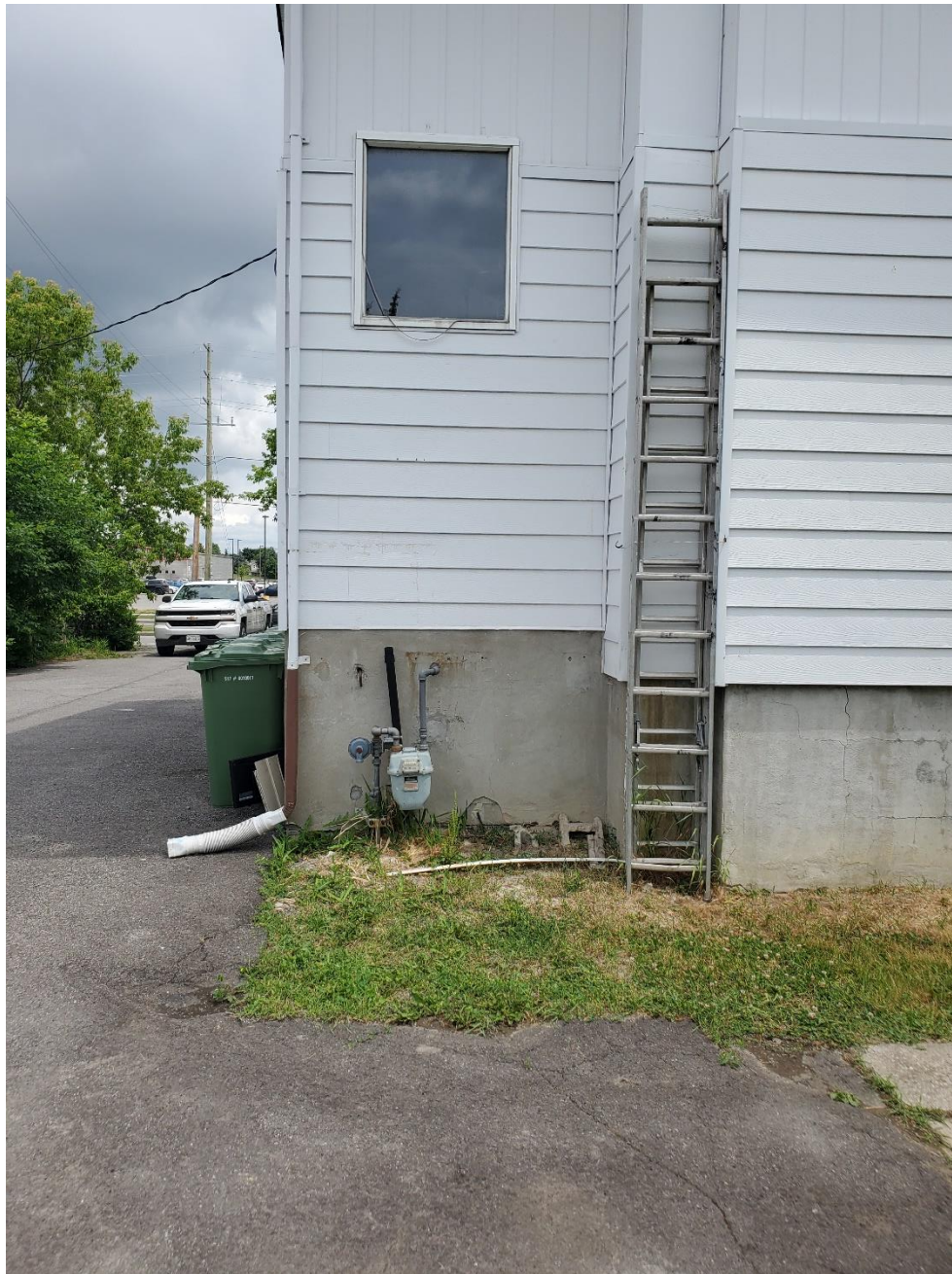
Photo 4: Facing east, gas enters the property from the west side of the building.
