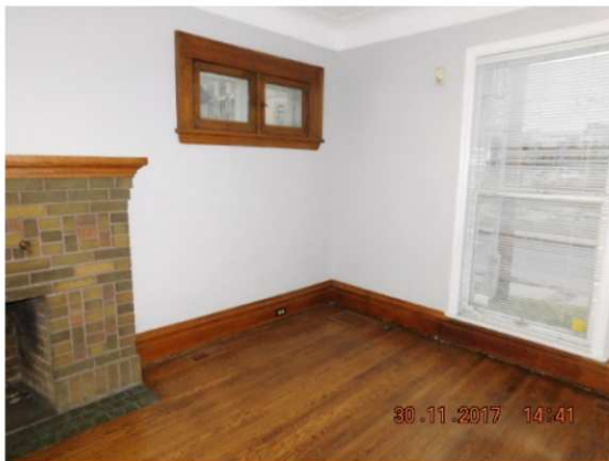
View of the first floor interior. Note the introduced window sill which extends almost to the floor, supporting the theory that the building originally had a more horizontal fenestration pattern similar to 263 McLeod. Note the original window to the right of the fireplace, and the simple casement detailing which is in keeping with a construction date in the 1925 – 30 period. The fireplace brickwork and pattern are also typical of the 1920 – 1930 period.
