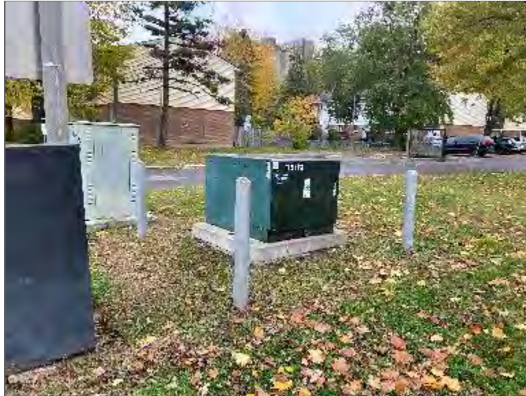
Photo 11 – Pad-mounted oil-cooled transformer located approximately 15 m northeast of the Phase One Property (PCA).
