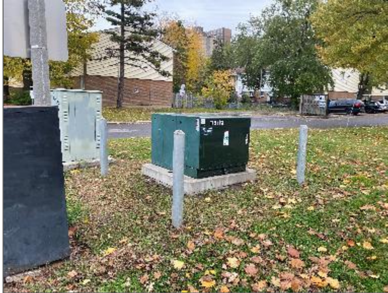
Photo 11 – Pad-mounted oil-cooled transformer located approximately 15 m northeast of the Phase One Property (PCA).
