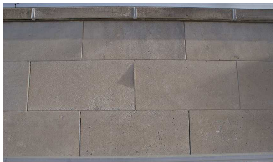
Figures 13: View of the Niagara limestone cladding above the Kent Street entrance. Note the variations in the material, coursing, and the windowsill course band the length of units corresponding with the cladding coursing. Mortar is missing from a number of joints. Source: Commonwealth 2023.
