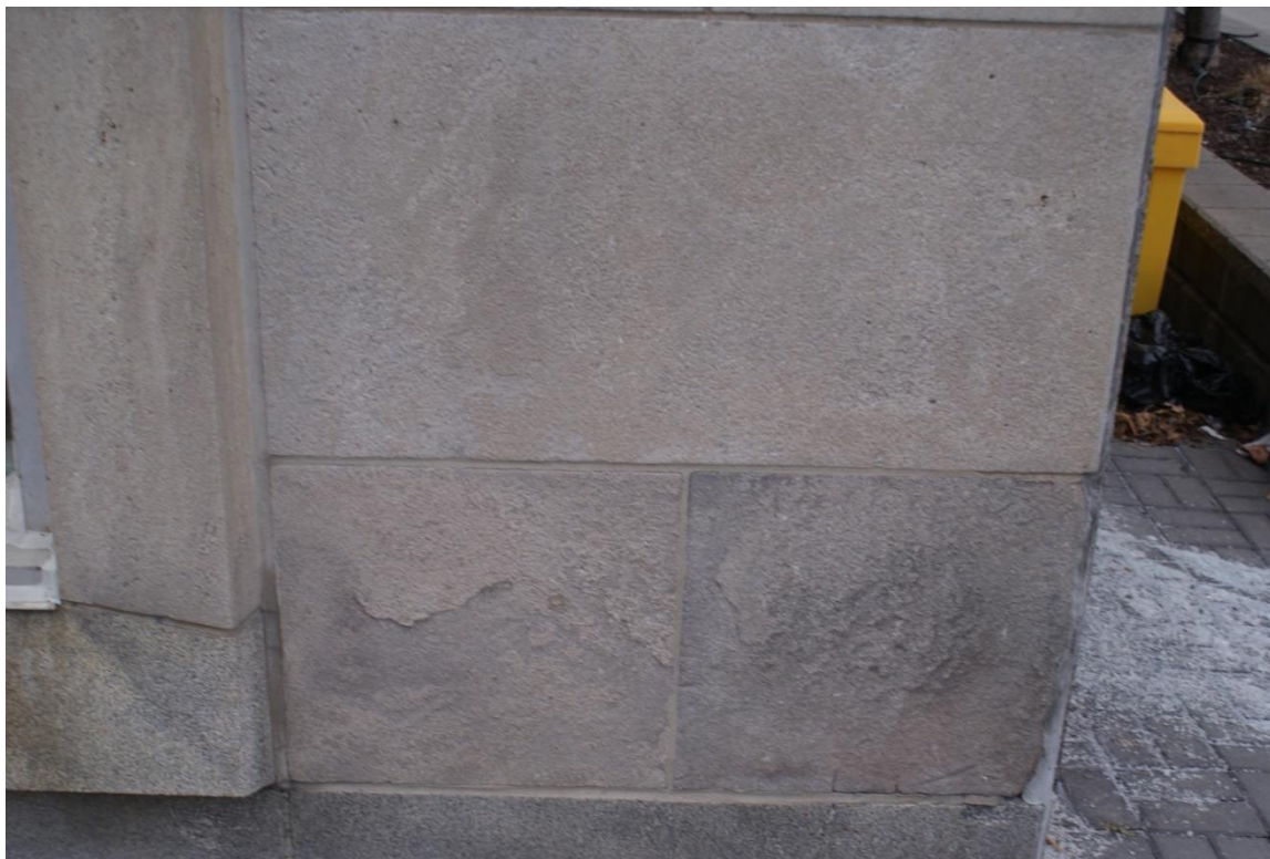
Figure 15: Detail view at the base of the wall at the south-west corner. The surface of the two Niagara limestone panels at the base of the wall are scaling due to de-icing salts. The granite plinth course is evident at the bottom of the photo. The Niagara limestone window surround is the vertical element to the left and a granite window sill/surround below. Source: Commonwealth 2022.
