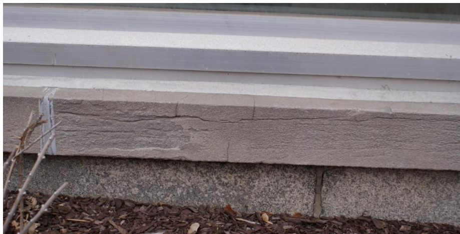
Figure 13: View of a deteriorated limestone windowsill and the granite plinth course below. The cleavage planes within the limestone sills are evident where the sawn surface has weathered. The cleavages planes follow the layers of deposition of the sedimentary rock. Source: Commonwealth 2022.
