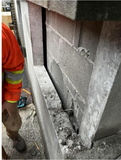
Figure 6: View of a test removal panel from a building at 100 Argyle constructed circa 1955 using a similar limestone cladding material as 359 Kent. The limestone cladding units are secured to the concrete block back-up wall with a single metal anchor centred on the width of the panel. Source: Heritage Grade Test Removal Report, 100 Argyle.
