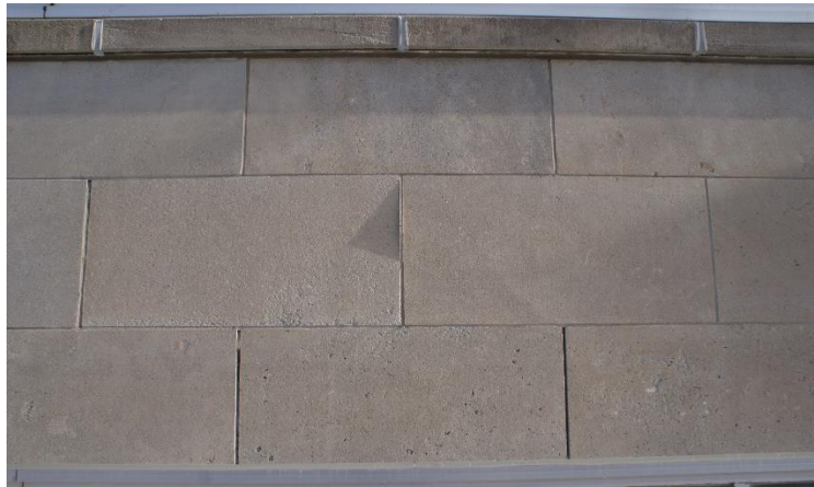
Figures 7: View of the Niagara limestone cladding above the Kent Street entrance. Note the variations in the material, coursing and the window sill course band the length of units corresponding with the cladding coursing. Mortar is missing from a number of joints. Source: Commonwealth 2023.
