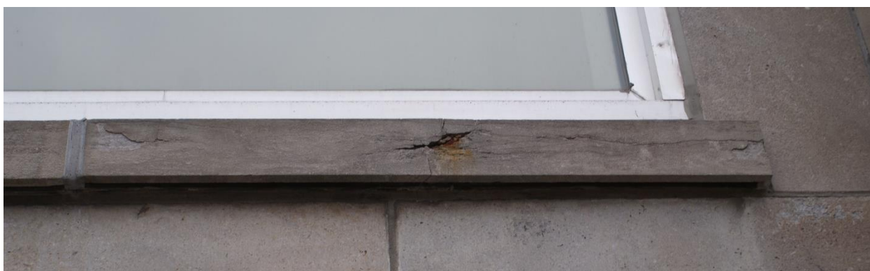
Figure 14: View of a deteriorated limestone windowsill. The cleavage planes within the limestone sills are evident where the sawn surface. The cleavages planes follow the layers of deposition of the sedimentary rock. Source: Commonwealth 2022.
