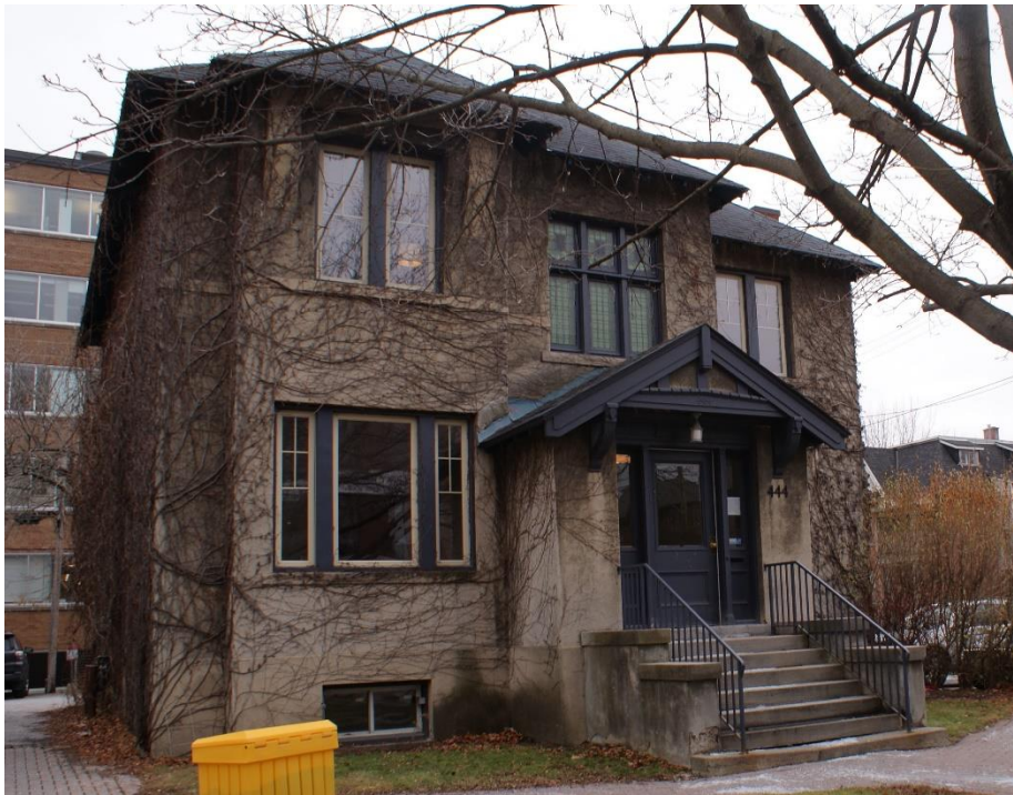
Figure 26: View of 444 MacLaren Street. The stuccoed exterior wall is covered in vines that should be removed before they have an adverse impact on the stucco finishes. Source: Commonwealth 2022
