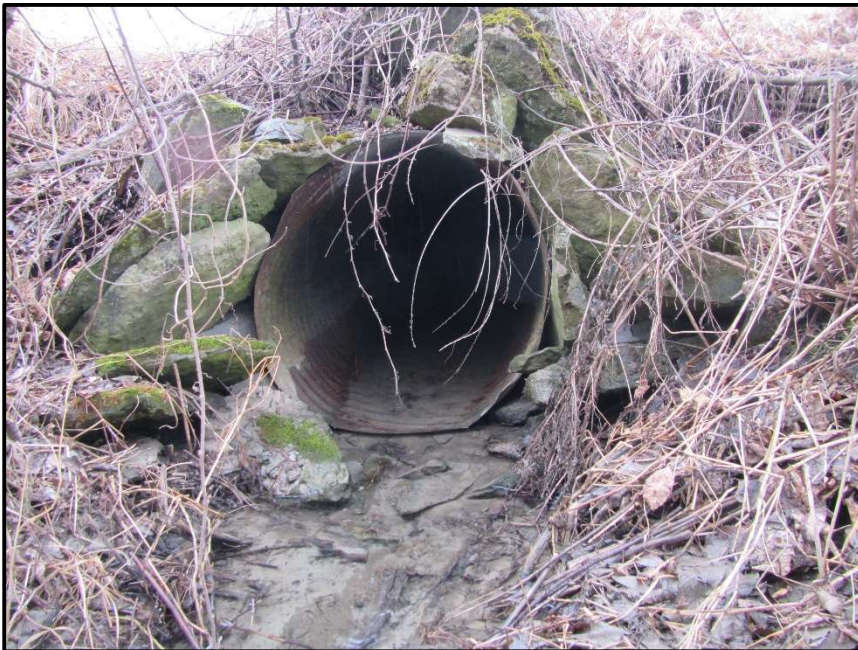
Photograph 6: 850 mm CSP culvert between the upstream and downstream portions of Survey Site #3 (March 24 th , 2021).
