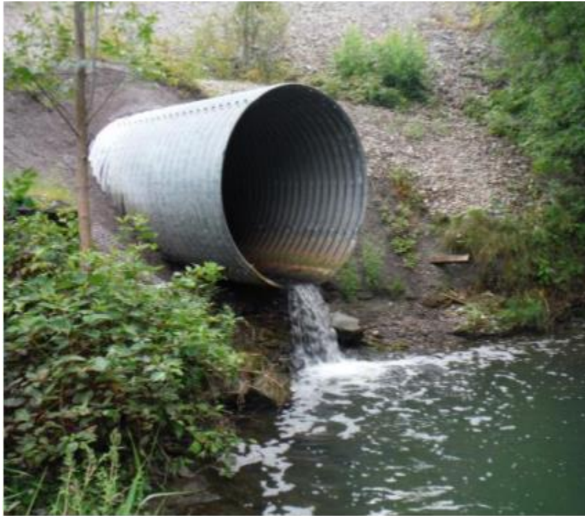
Photo 2: Perched culvert that conveys flow of Stillwater Creek under the Beachburg railway (RVCA, 2015)
