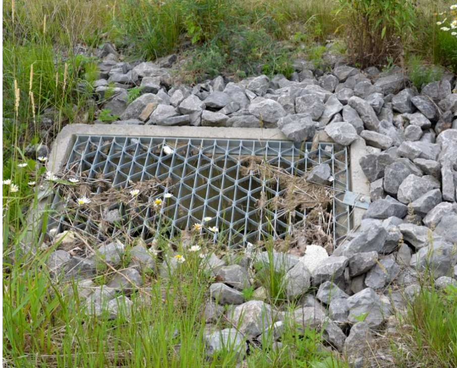
Photo 3 – Channel ends at a storm grate on the north side of Donald B. Munro Drive. View looking west
