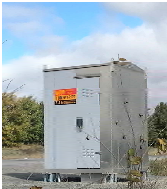
Photo 28 – A transformer associated with the Via Rail visible along the northern Site boundary at 4375 McKenna Casey Drive.
