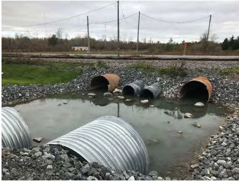
Photo 21 – Drainage pipes, railway line and McKenna Casey Drive to the north of the Site at 4375 McKenna Casey Drive
