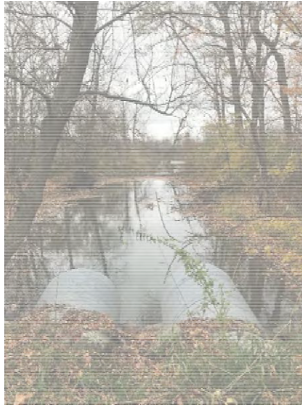
Photo 5 – Discharge pipes into river tributary on the south-east corner of the Site at 3305 Borrisokane Rd
