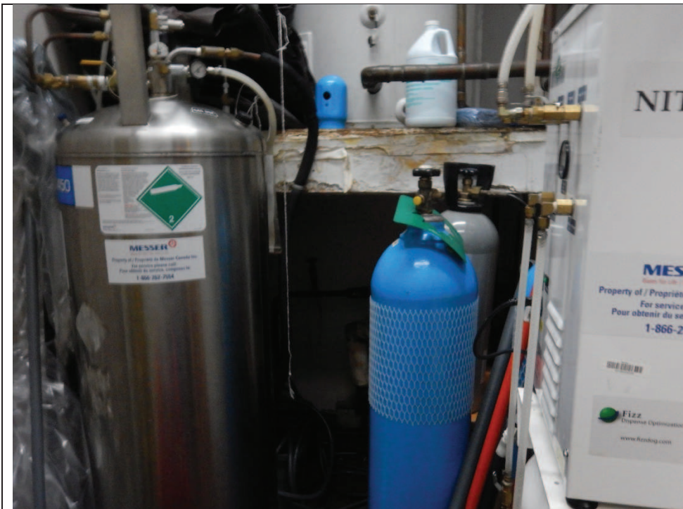
Photo 24: View of the chemical storage room for the Montana's, commercial size cleaning chemical - 2021
