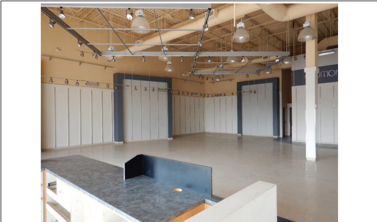
Photo 6: Interior of the vacant portion of the commercial retail space on the Phase One Property (facing west) - 2021
