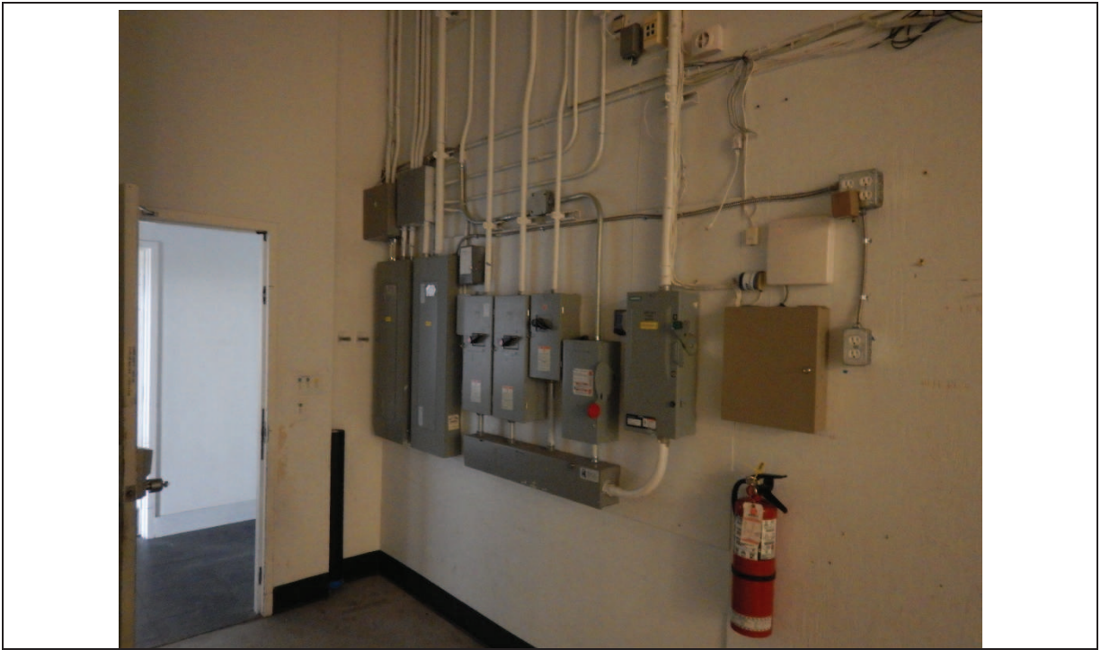
Photo 7: Typical electrical service in the vacant commercial retail space on the Phase One Property
