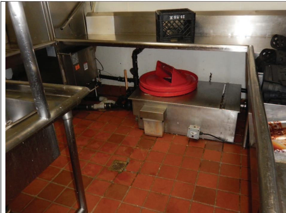
Photo 25: View of the grease trap in the Montana's
