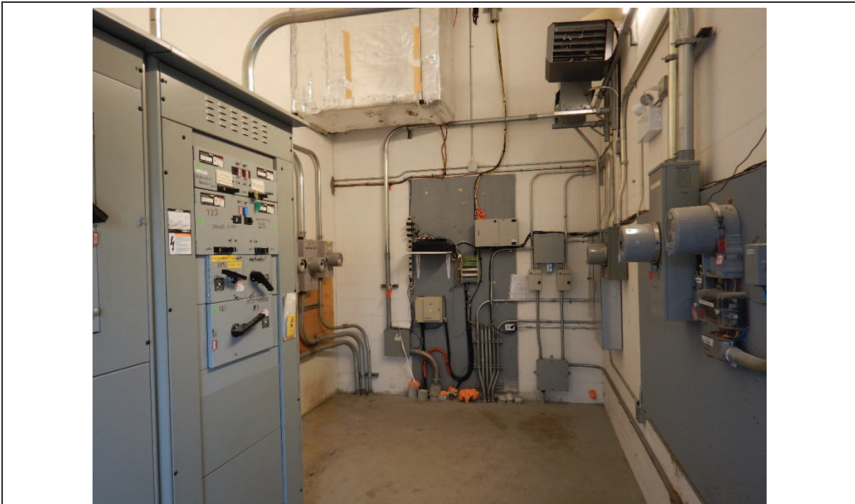
Photo 10: Transformer room for the vacant commercial retail space and Cineplex on the Phase One Property
