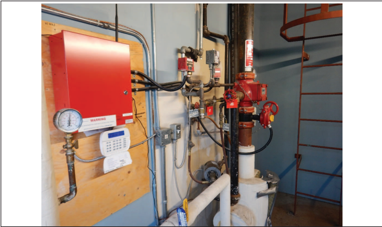
Photo 9: Water service in the vacant commercial retail space on the Phase One Property
