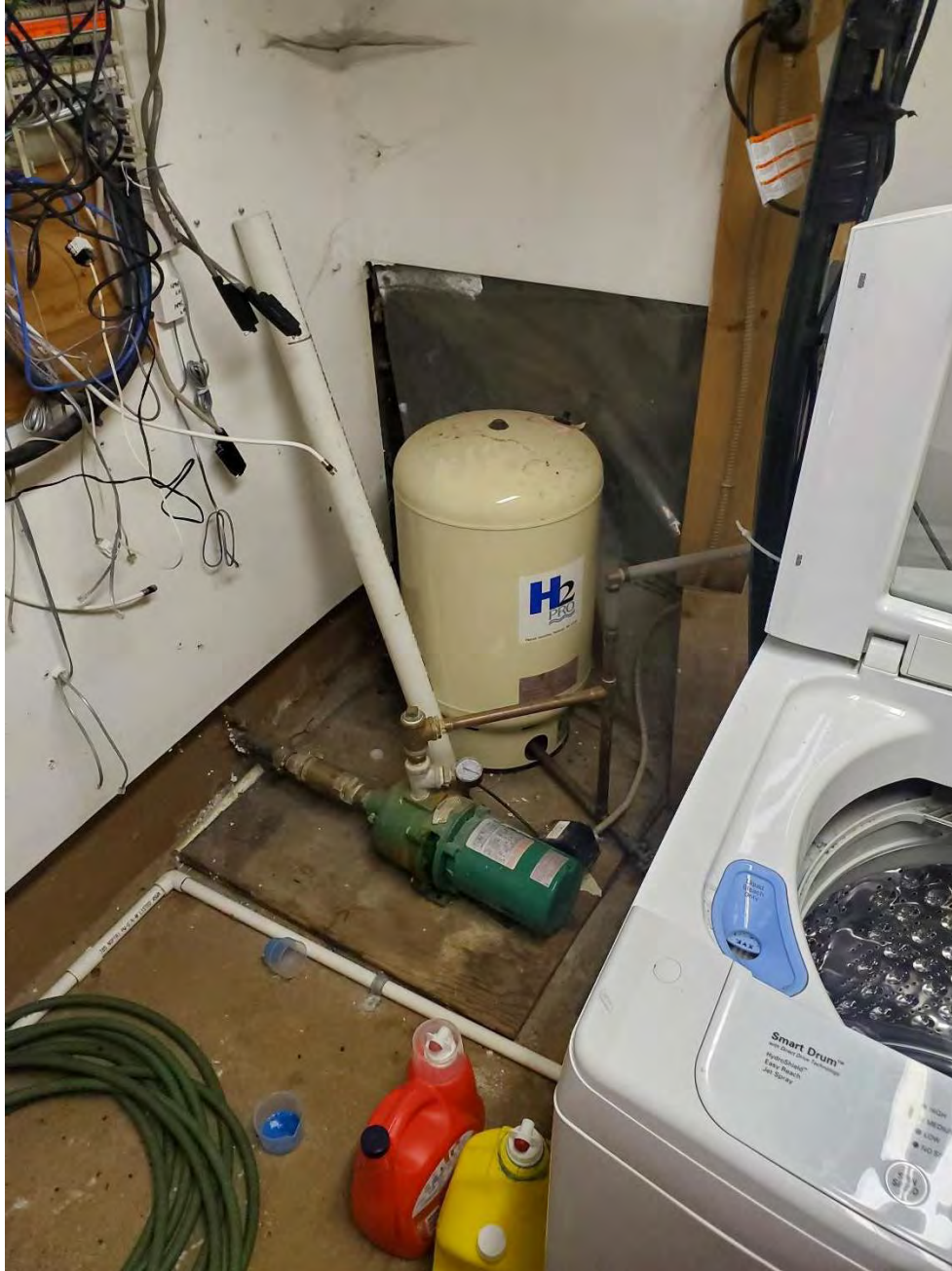
Photo 3: Facing northwest, sump pump and a well tank located in the basement of the site. The site is serviced by a potable water supply well.
