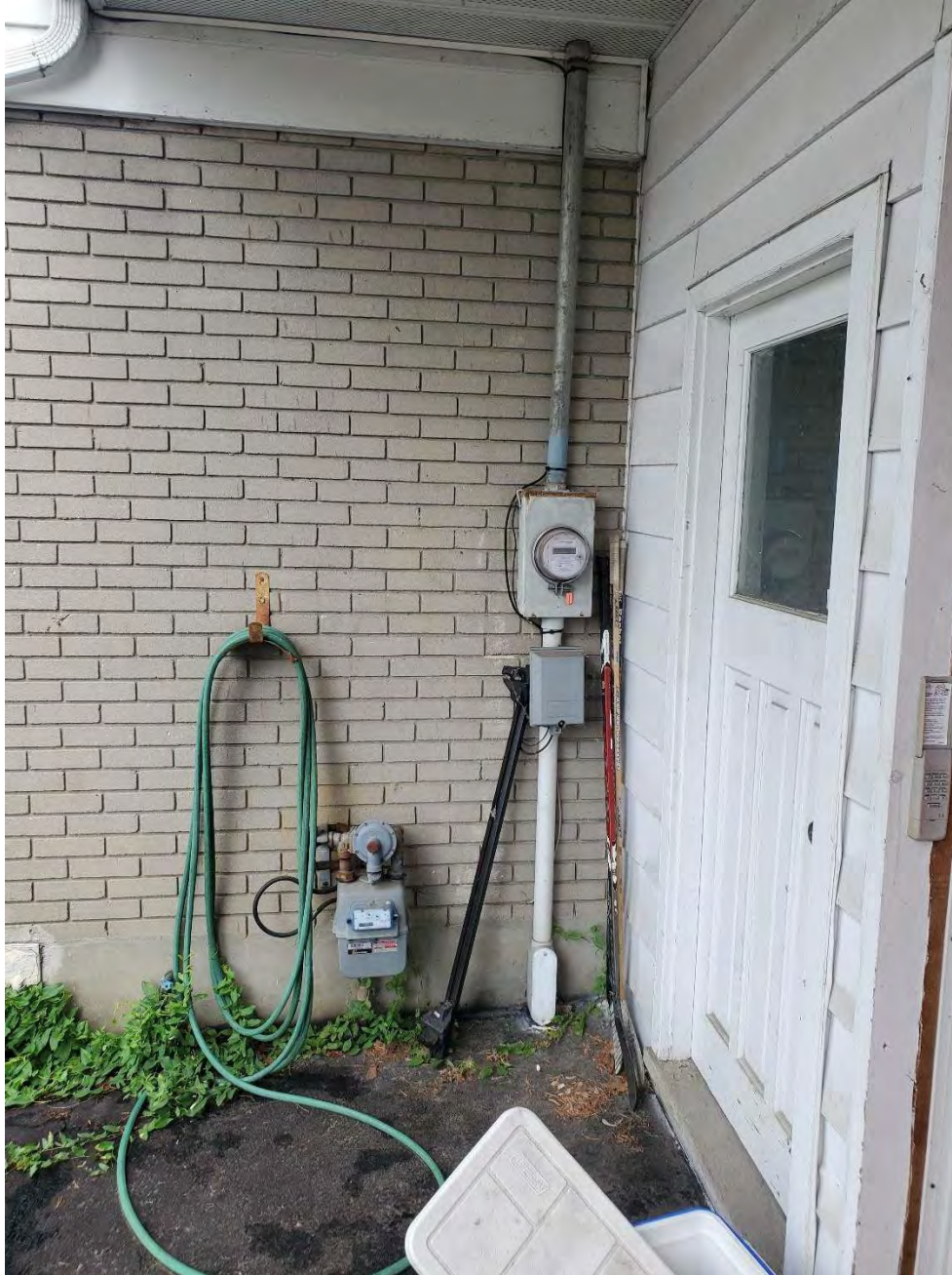
Photo 2: Facing northwest, Gas and overhead hydro lines enter the property from the east side of the building.
