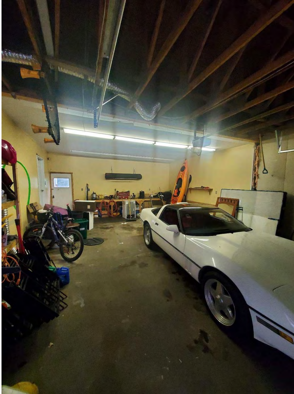
Photo 4: Facing northeast, the attached garage located on the east side of the building had minor oil stains present
